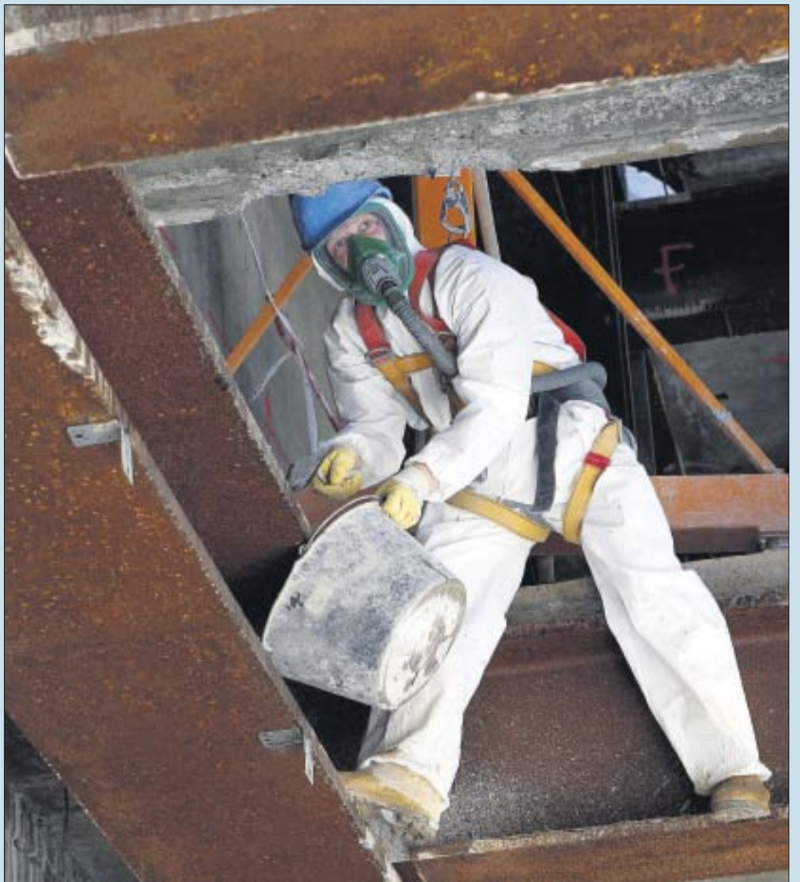
DANGEROUS WORK: Removing asbestos is a major hazard for ship recyclers.
