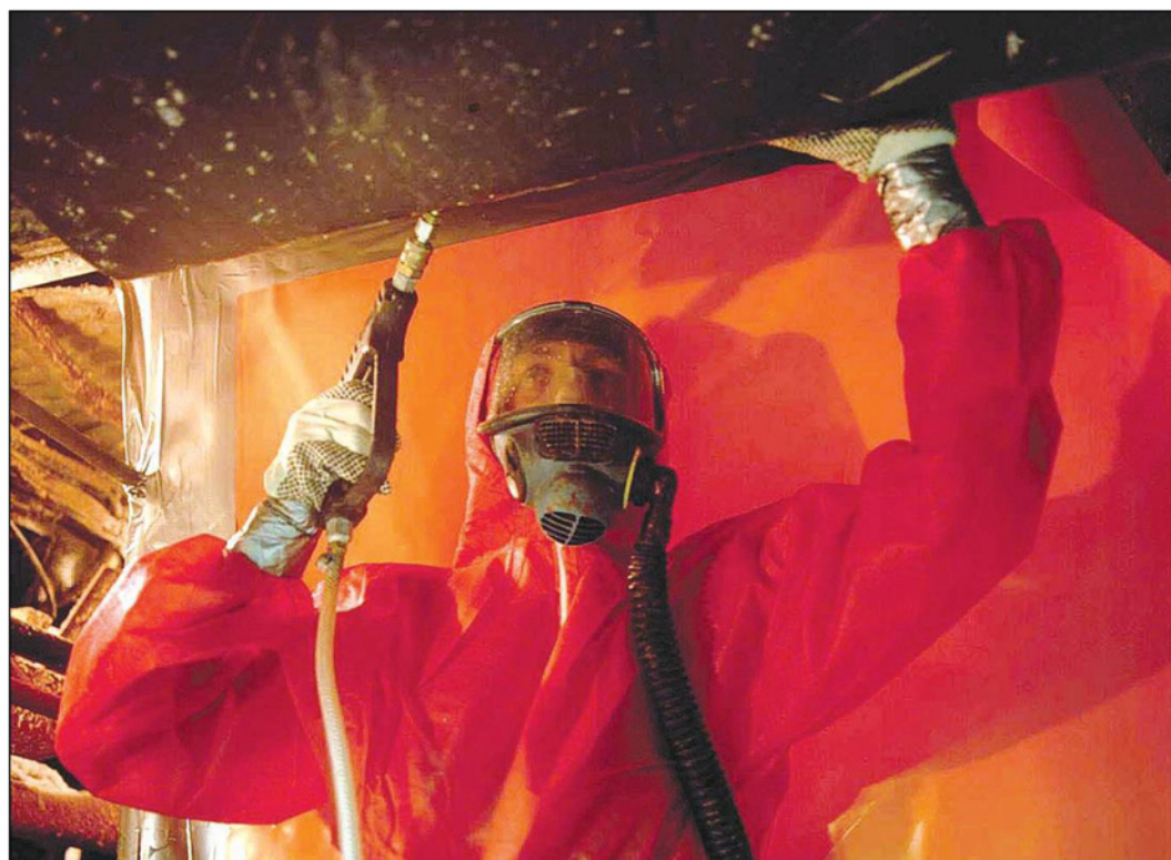
Removing asbestos: despite its use technically having been banned since 2009, only five of the six types are covered by law.
